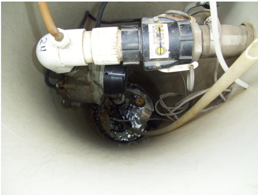
Figure 14: Inside water sampling sump
